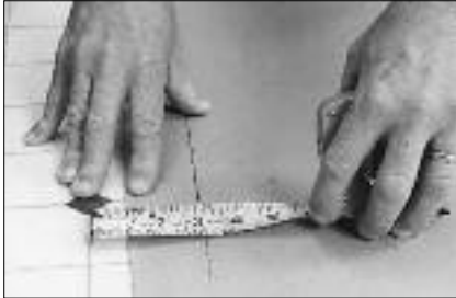
After you have transcribed the entire area to the paper, carefully remove the pattern and place it on the resilient floor covering to be used. Take the time to square the pattern to the resilient floor covering using a tape measure or ruler and be sure to center the pattern.
