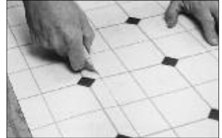
Follow the pencil marks on the surface of the resilient with a knife or scissors. Use caution so you don't damage the underfloor you're working over. A hookblade utility knife may make this easier.
